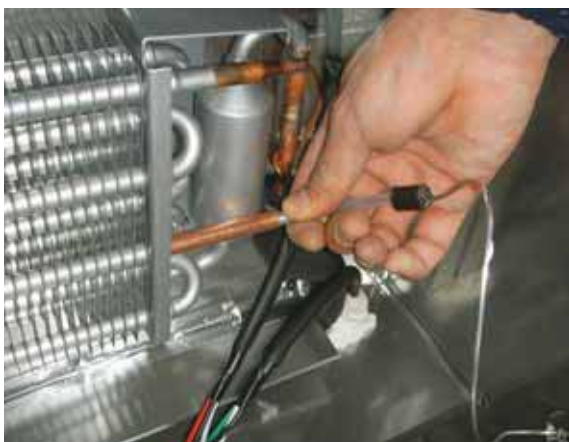
TEMPERATURE CONTROL & EVAPORATOR
