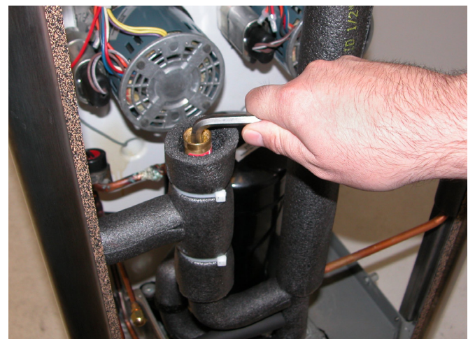
Figure 3-8 Hot Gas Bypass Adjustment
