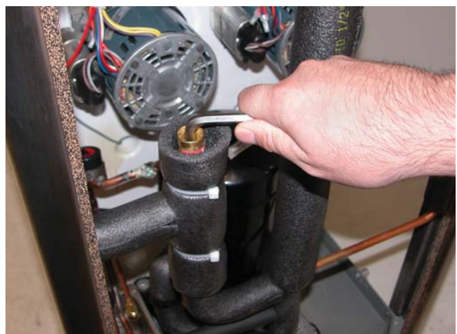
Figure 5-10 Hot Gas Bypass Adjustment
