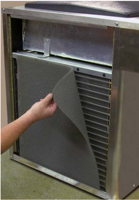
Figure 3-8 F112 Condenser Filter Removal
