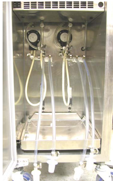
Figure 2-7 Completed BCS Hose Assembly
