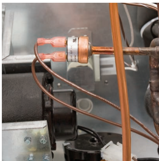
Fan Pressure Control, must CLOSE to operate fan motor.
