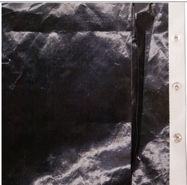
BELT IS TORN AND FOLDED. REPLACE BELT.
