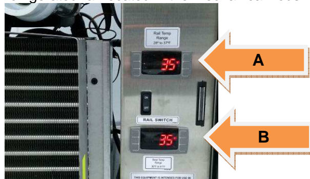
Figure 1 illustrates the inside of the mechanical housing behind the louvered panel. Item A is pointing out the temperature control for refrigerated rail. Item B is pointing out the temperature control for the refrigerated base.
