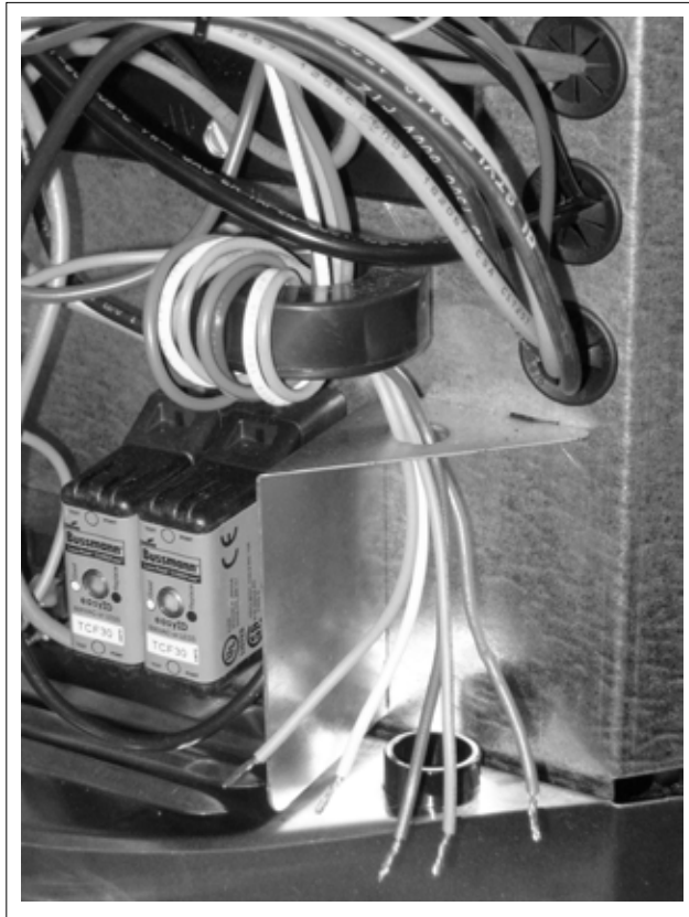
Figure 5. Low Voltage Compartment Control Wiring Connections
