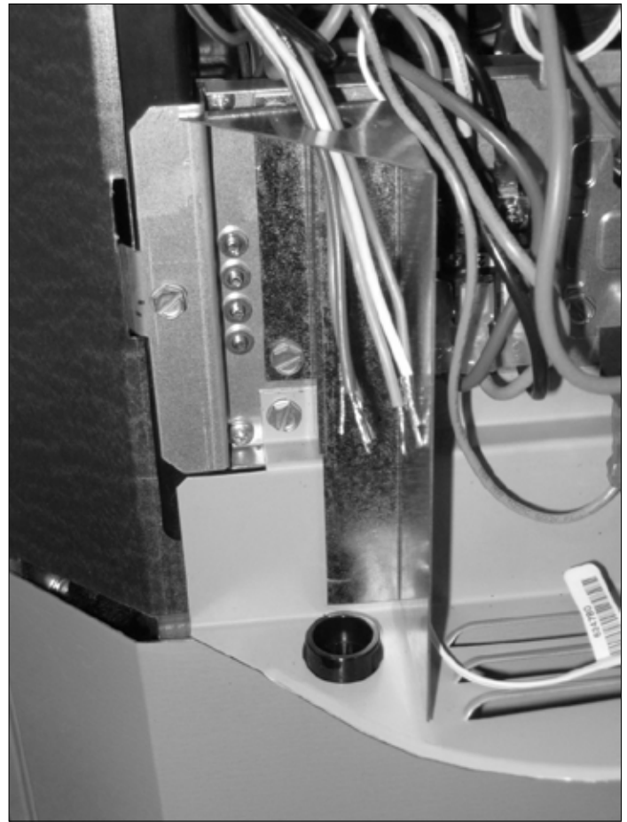
Figure 4. Low Voltage Compartment for Control Wiring
