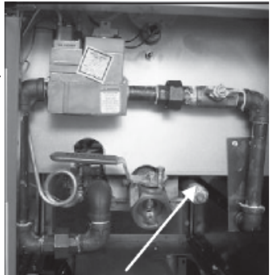
A manometer or water column pressure gauge meter is connected to the manifold here.
