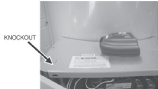
Figure 16. Location of Communications Wiring Knockout
