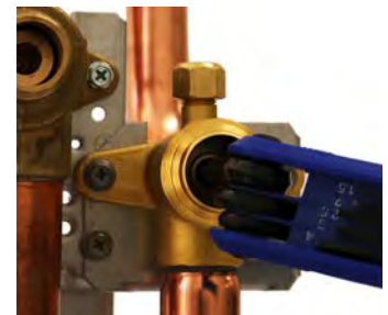
Opening the Service Ports.
