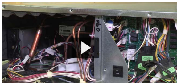
Demonstration of Control Board Replacement
