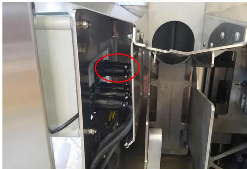
Figure 67. Location of Safety Cables
