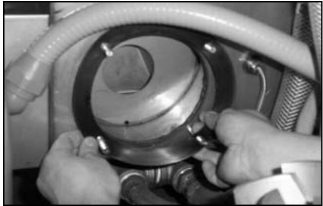
Removing the pump gasket
