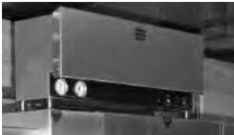
Control Box Gauge Location
