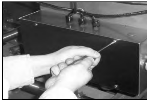
Removing the heater box cover
