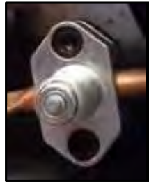
refrigeration line tapping valve
