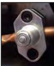
refrigeration line tapping valve
