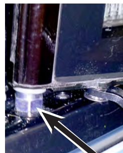
(Not Properly Engaged in Hinge Plate)
