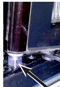
Not Properly Engaged in Hinge Plate
