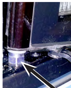
(Not Properly Engaged in Hinge Plate)
