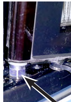
Not Properly Engaged in Hinge Plate
