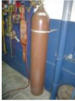
DRY NITROGEN EQUIPMENT
