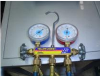
MANIFOLD PRESSURE GAUGES
