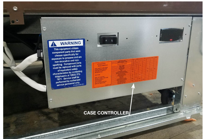
Fig. 6 Case controller location
