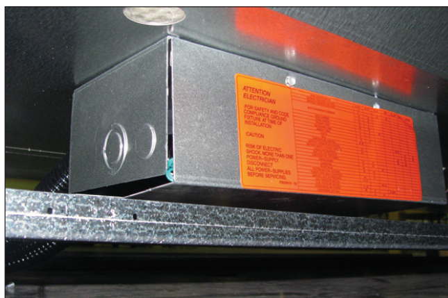
Fig. 14 Junction box beneath case
