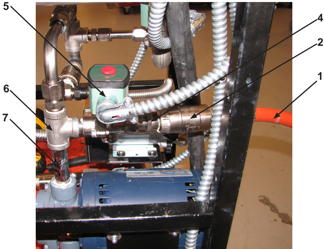
Bulk Dispose - EEE-181
