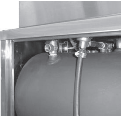
One of the pressure relief safety valves is located on the top left rear of the boiler.
