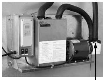
Connect glycol recirculating line from pump outlet 3/8" barb fitting to the beer line set.
