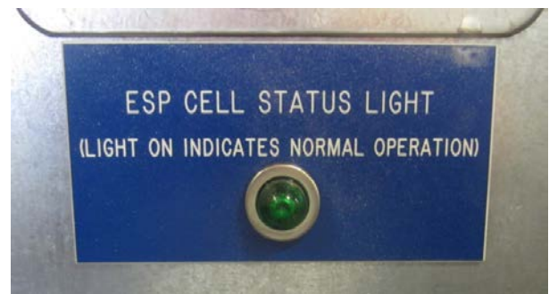
Figure 3-4-4 ESP Cell Status Light Located on Wash Control Cabinet
