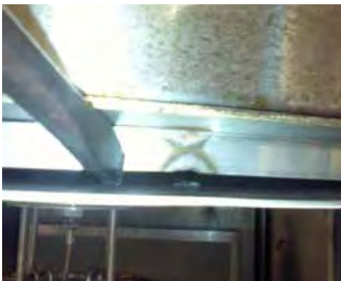
Example of broken weld
