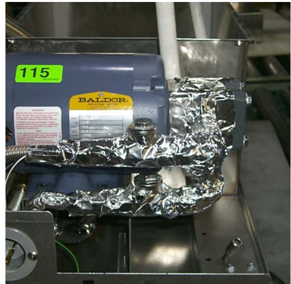
Heater strip installed [115V PF50 (Return/Suction)].
