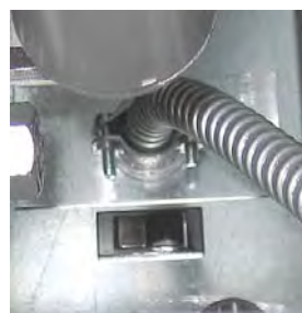
Figure 14 (Rear view of Control Box)
