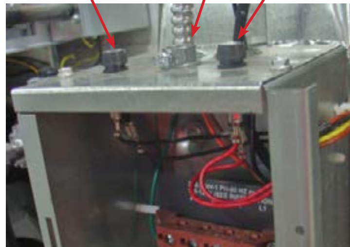
Control Protection Fuse 2.5 Amp 14 1 14 Ignition Upper Pocket Protection Fuse 1.5 Amp
