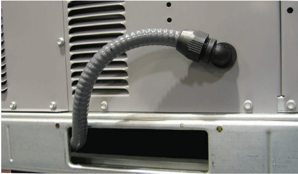
Fig. 4 - Detail showing drip loop to prevent water from collecting in liquid tight conduit.
