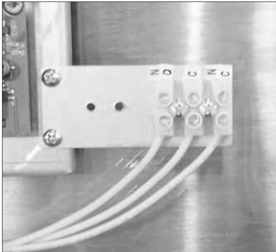
The Low temperature interlock block is located on the right-side of the booster cabinet interior.
