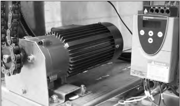
Variable Frequency Drive (VFD) shown with the Conveyor Drive Motor
