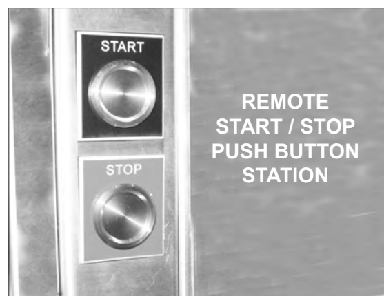
A Remote Start/Stop Station is located on the load-end of the dishwasher.
