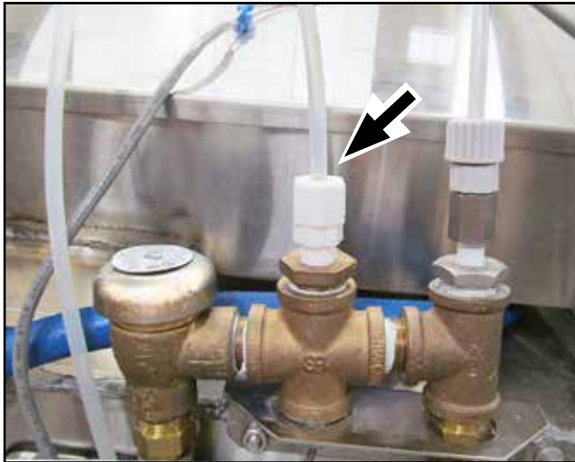
Fig. 20 - Rinse aid injection point
