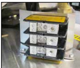
Fig. 3 - Booster terminal block
