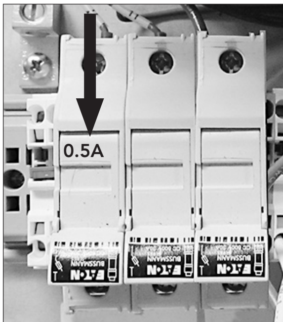
Fig. 8 - Connection is located inside the top control cabinet.
