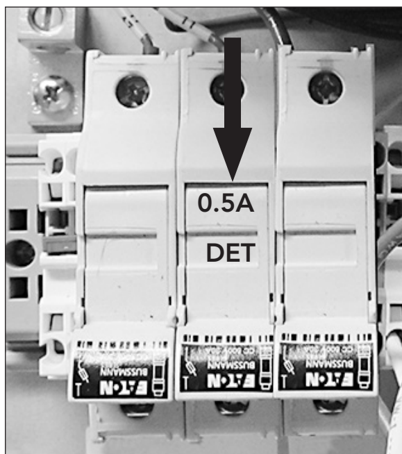
Fig. 10 - Connection is located inside the top control cabinet.
