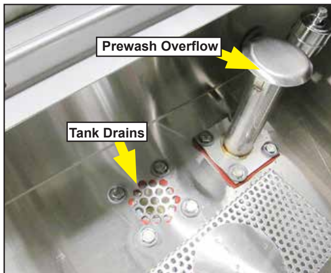
Fig. 72 - Tank drain prewash overflow
