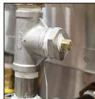
Fig. 22 - Final rinse manifold
