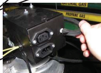
Pressure switch tubing
