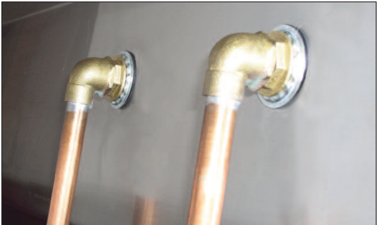
View From Back of Sink
