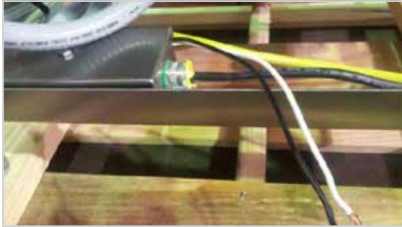
Power junction box for incoming 120v power
